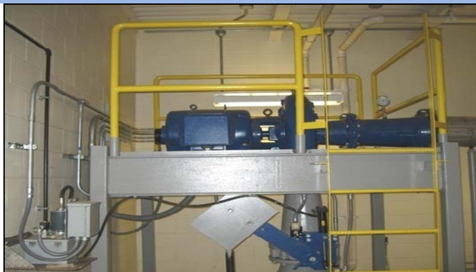
Turbine unit at control valve site
