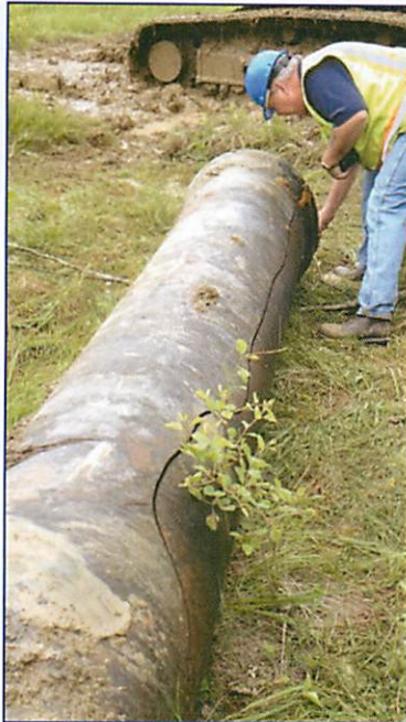
Failure of an old water main in May 2014 and the flooding that resulted (shown in the picture below).
