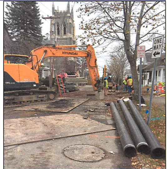
THE WORK BEGINS —State Street at French Street, fall 2017. Plans for 2018 include work on lower State Street, French Street, and Exchange Street.
