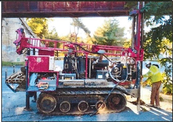
LEDGE PROBE—A contractor checks for underground ledge along the planned path of a new water line on Main St. in Bangor.
